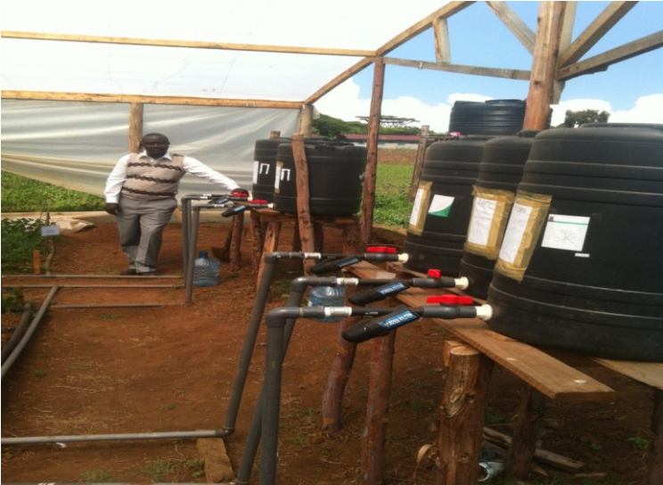
Figure 3.5 Main and treatments tanks
